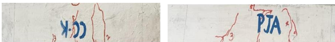
Figure for Crack pattern for 0% & 20% PJA beam
